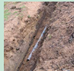
When will this pipe be connected?
