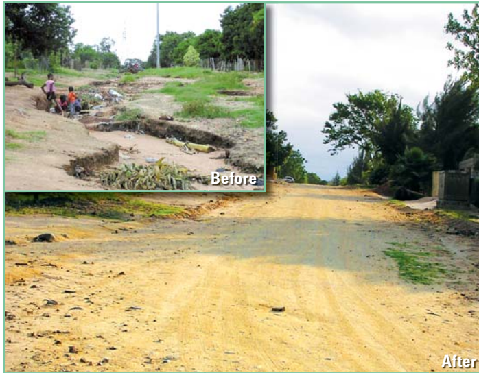
Left: Figure 4.13 A road that had not been maintained for years. Residents had to park their cars at the end of the road
