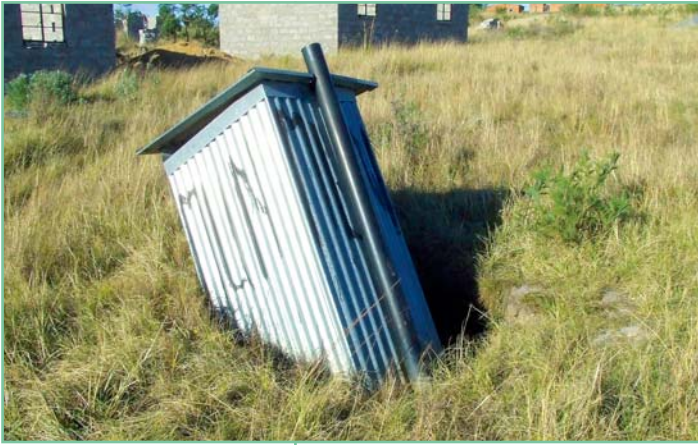
Figure 4.5 Inadequately lined pit
