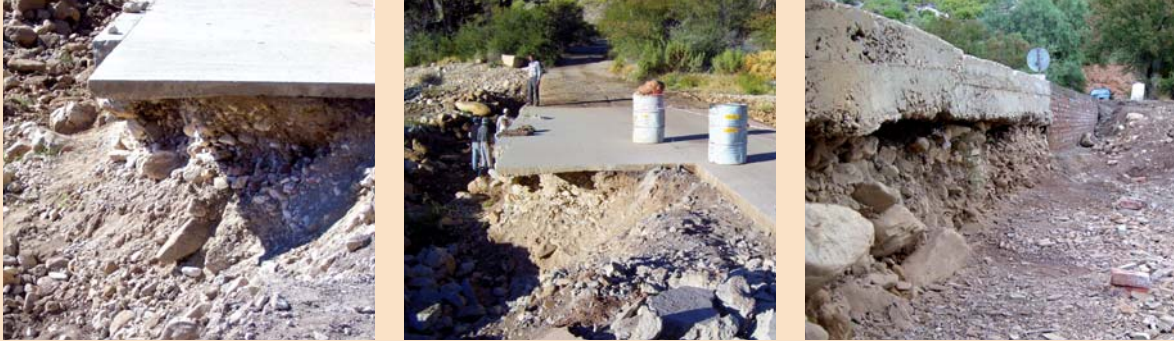
Blocked low-level bridge resulted in slabs being washed away and the remaining support being undercut
