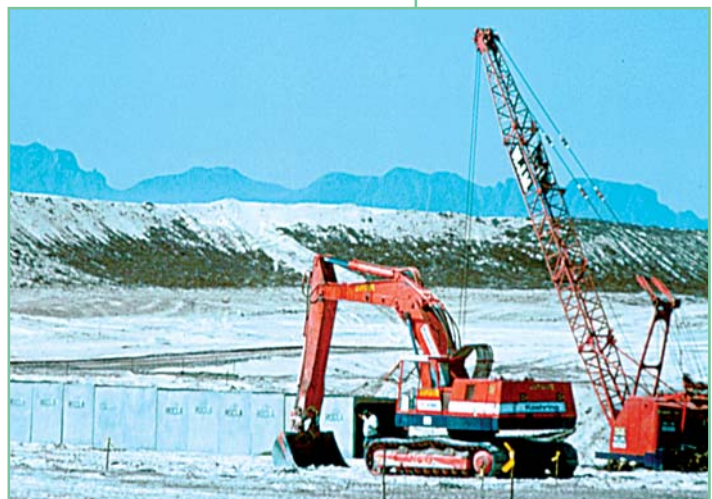
Figure 2.12 Constructing a two-metre deep box culvert stormwater drain under Mitchells Plain to allow for its long-term development, 1979
