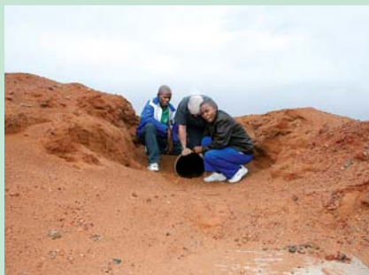
Where on earth is this pipe going?
