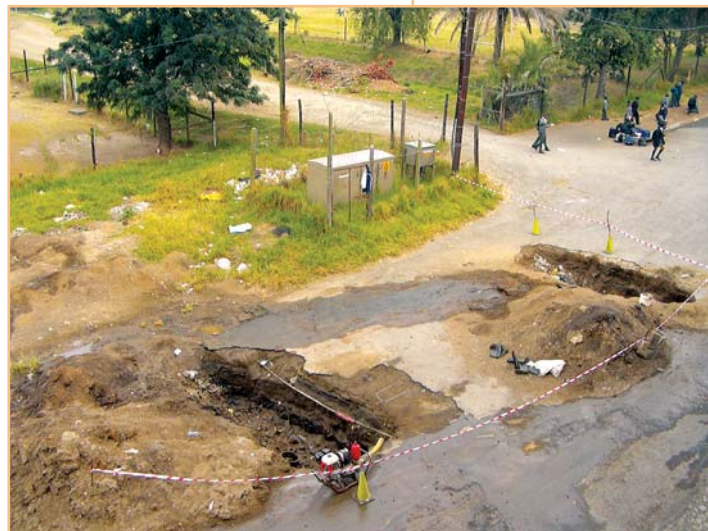
Figure 5.11 Reinstatement required by one municipality after excavations had been carried out by the water service provider. Lack of coordination and resources resulted in the excavation remaining open for many months
