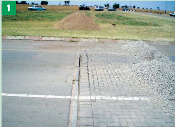
Broken paving in intersection
