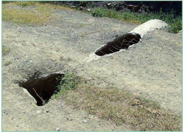
Figure 4.6 Pipe laid too close to the surface
