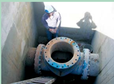
Air valve on bulk line
